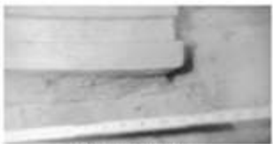
FIGURE 2.05 Crack between two welds
