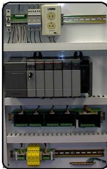
FIGURE 11.3: CONTROL PANEL WITH PLC (GREY ELEMENTS IN THE CENTER). THE UNIT CONSISTS OF SEPARATE ELEMENTS, FROM LEFT TO RIGHT; POWER SUPPLY, CONTROLLER, RELAY UNITS FOR IN- AND OUTPUT
